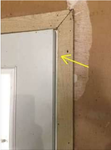
Photo 4-3 Door binds at top of jamb and does not close easily.
