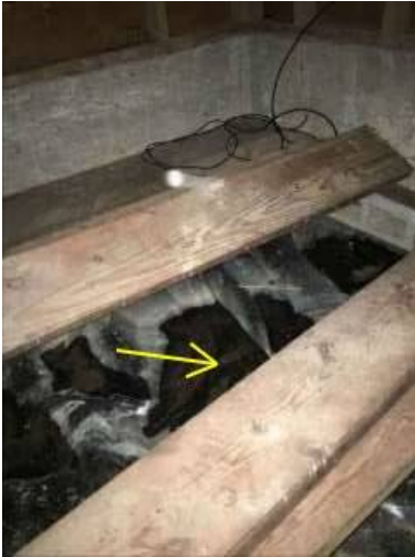
Photo 18-3 Standing water and sediment deposits.
