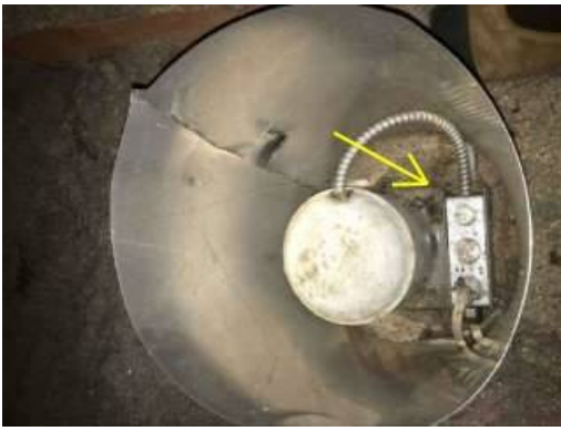
Photo 10-3 Baffle, which holds back insulation from the heat of the light fixture, and gaps around fixture may be providing a path to the attic for warm moist air (there were five of these observed in the attic space).
