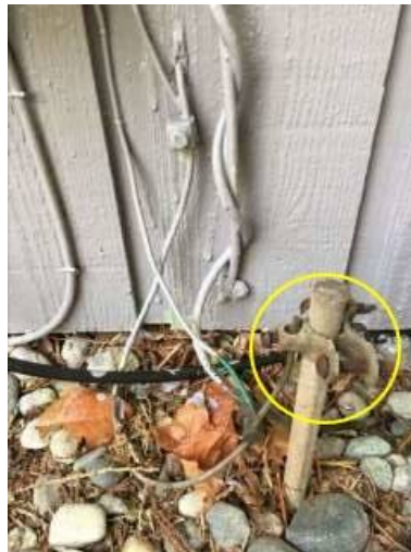
Photo X-18 Grounding rod connected to electrical panel.
