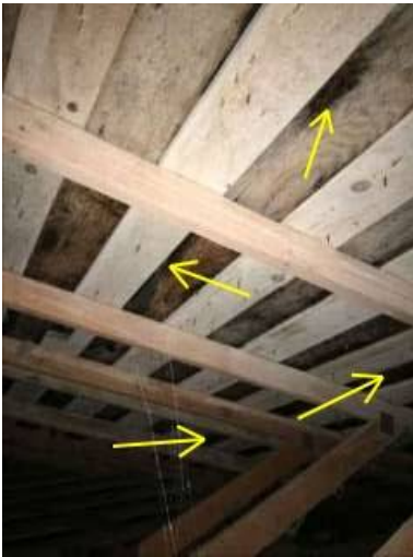
Photo 10-1 Arrows indicate locations of observed condensed moisture. Also apparent is a patina of white fungal growth. This condition was observed in a wide ranging area above the attic access hatch.
