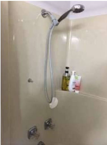
Photo 15-1 Leak in p-trap beneath this fixture.
