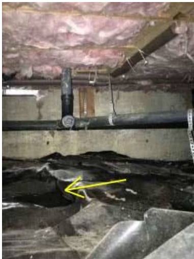
Photo 15-3 Puddle left by leak.
