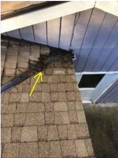
Photo 4-1 Exterior door to garage and flashed valley, clogged with tree debris, above downspout.
