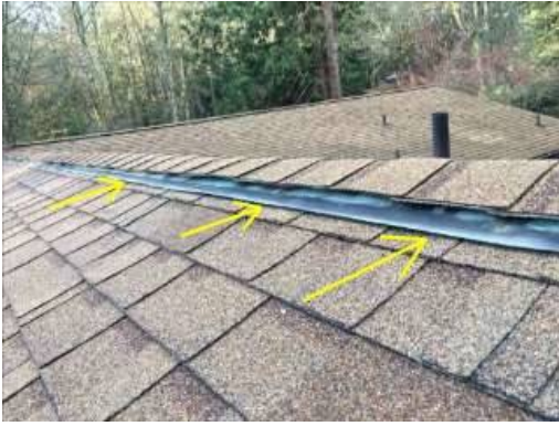
Photo X-11 Zinc strip at ridge vent to inhibit moss growth.
