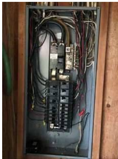
Photo X-20 Cover off electrical panel.
